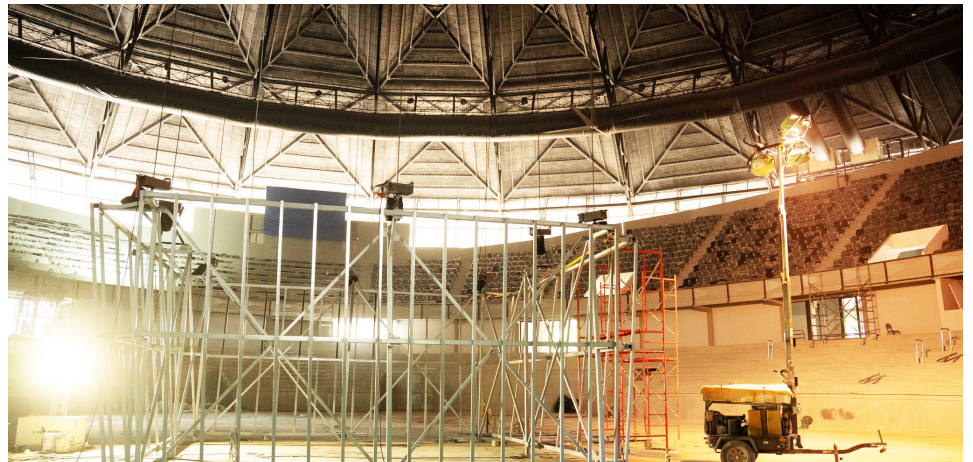
A view of the work being carried out at the Virgilio Travieso Soto Sports Palace.
